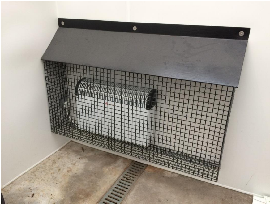
Electric heater with mesh protection and sloping metal cover
