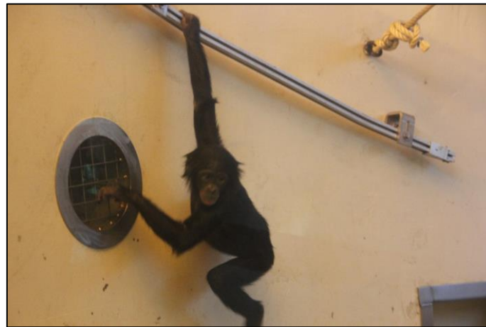
Figure 37: Air vent installed to allow air circulation between adjacent enclosures also when the full slides between the enclosures are closed off (Apenheul – Jeroen Stevens).
