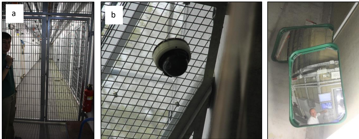
Figure 59: Safety measures to increase visibility or safety in service corridors. a: safety doors (Wilhelma Zoo Stuttgart–Jeroen Stevens); b: safety cameras (Wilhelma Zoo Stuttgart–Jeroen Stevens); c: Safety mirror to avoid blind angles (Wilhelma Zoo Stuttgart–Jeroen Stevens).
